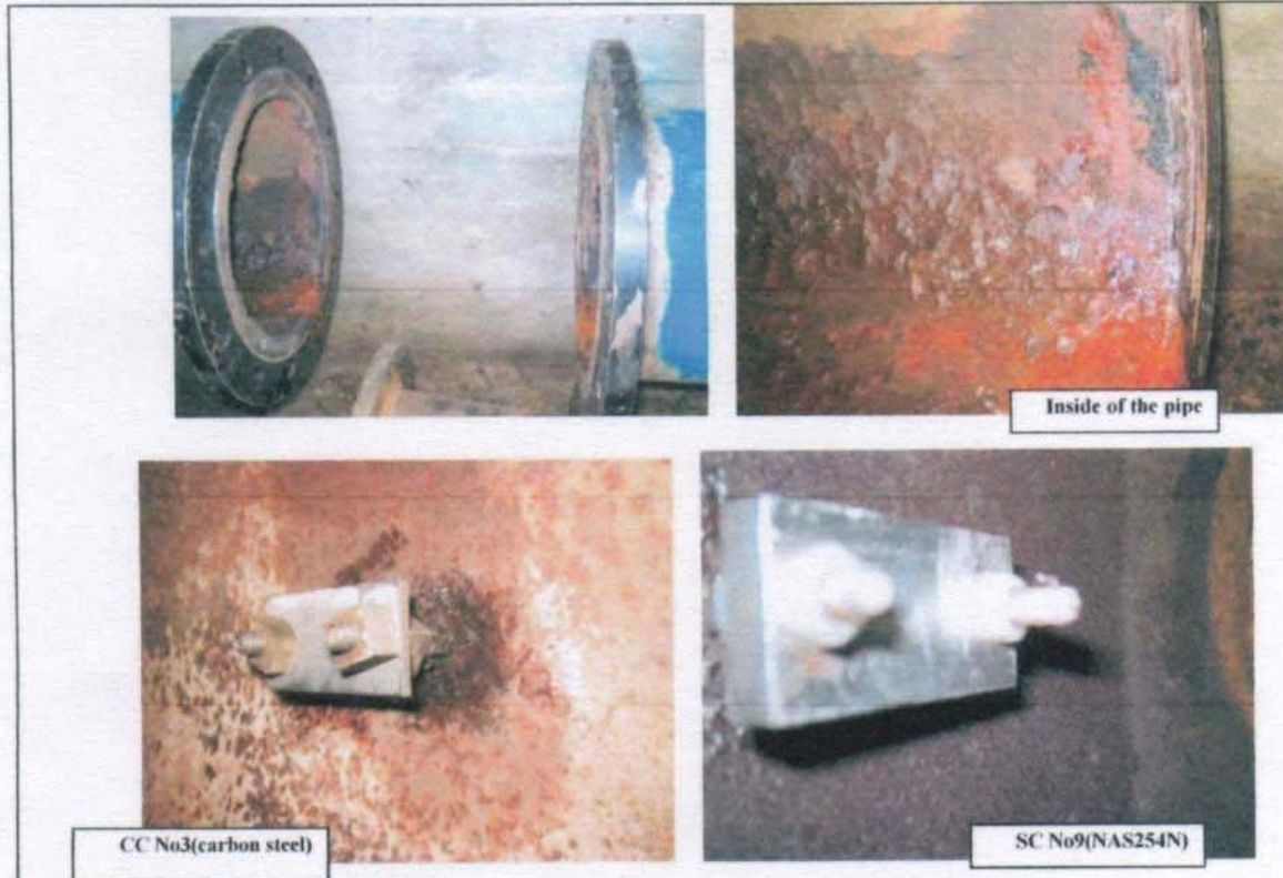
Fig.(6): Shows the installation of the Corrosion Coupon and Scale Coupon in Position No.3(10 inch)
